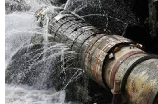
Low efficiency, Leakages on distribution networks
