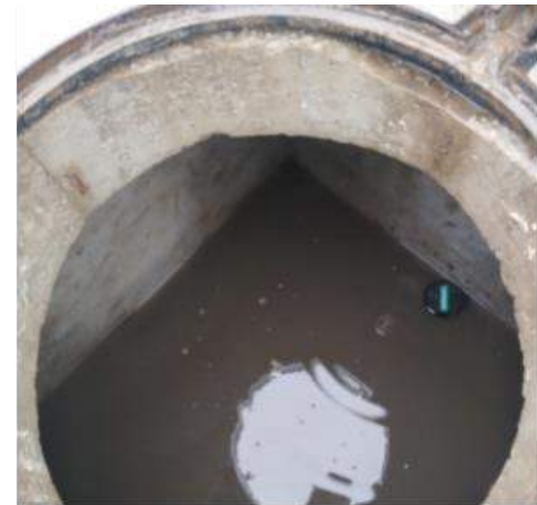
Flooded Flow Meter housing
