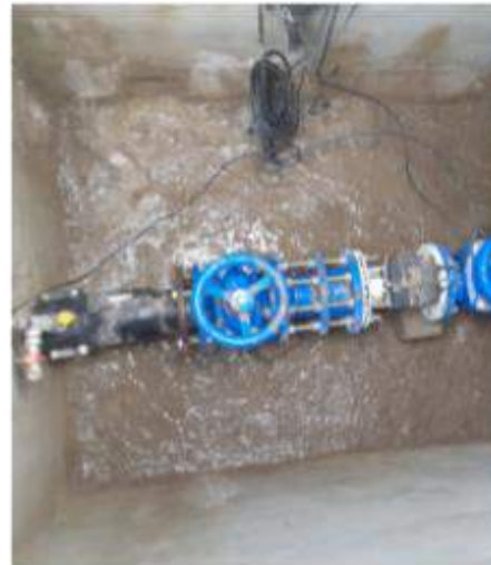
Flow Meter housing
